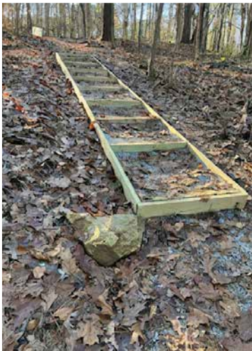
Standing at the bottom of the steps looking up the hillside from the creek.
